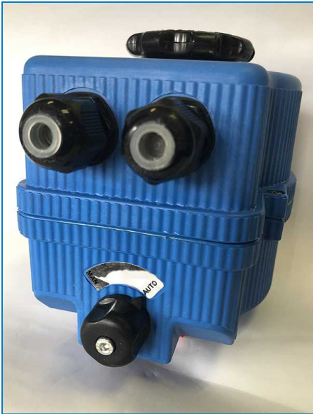
Purge valve actuator position "AUTO"
